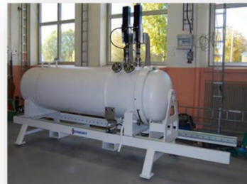
Mounted on Support Structure
