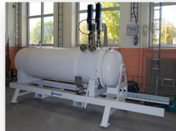
Mounted on Support Structure
